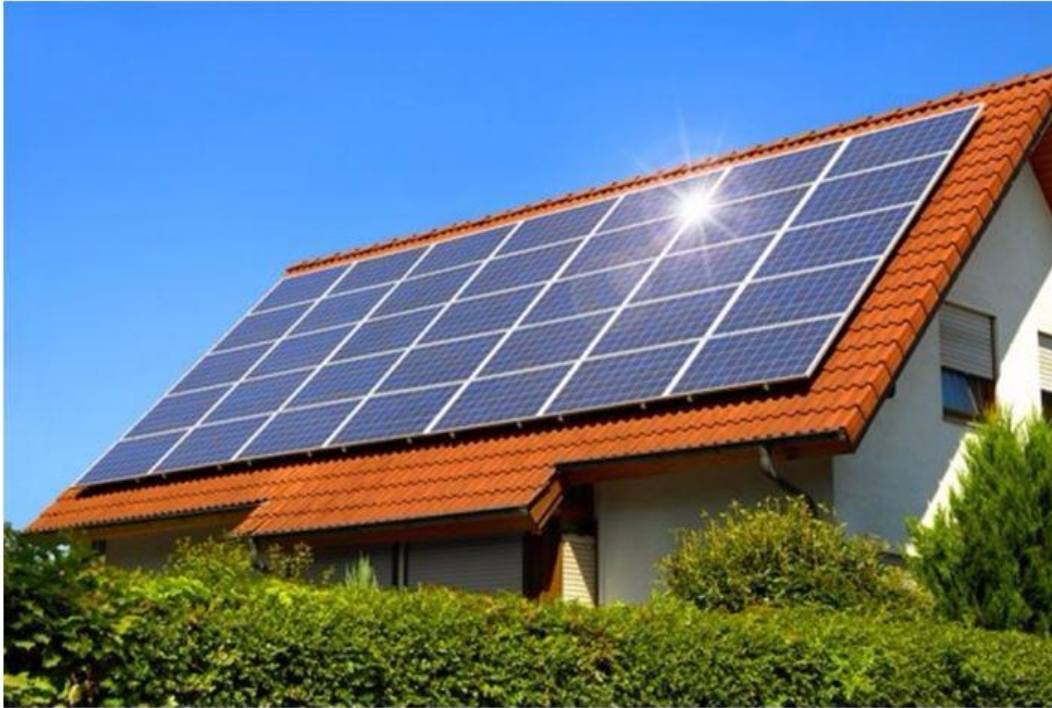
Rooftop solar panels
