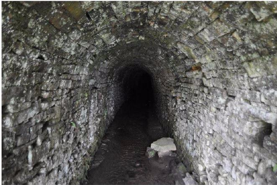
Horse level Adit in the abandoned lead mine, Nenthead, County Durham, UK
