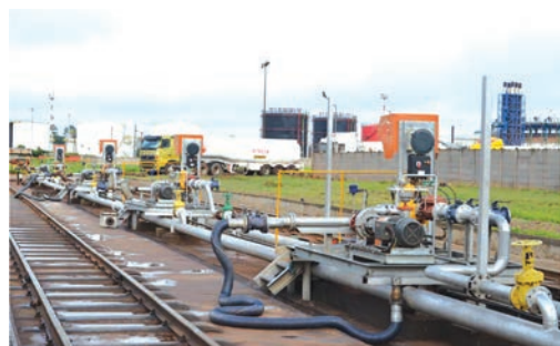
Figure 9.6 TAZAMA oil pumping station
