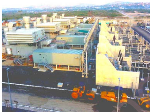
Figure 8.6 Natural gas plant at Kinyerezi 1, Dar es Salaam
