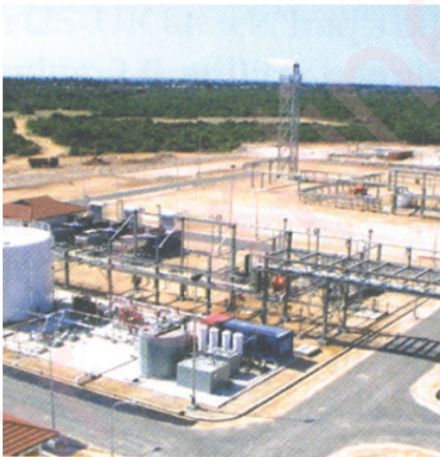
Figure. 5.5 Songosongo gas plant
