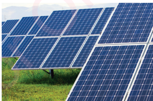
Figure 2.2 Solar panels for electricity generation
